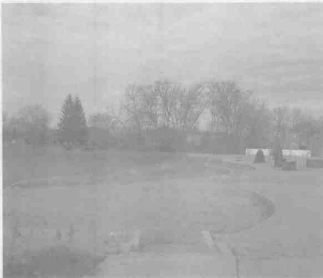
The recently completed stormwater basin at the Our Lady of Ransom parish grounds | IGOR STUDENKOV/FOR PIONEER PRESS
