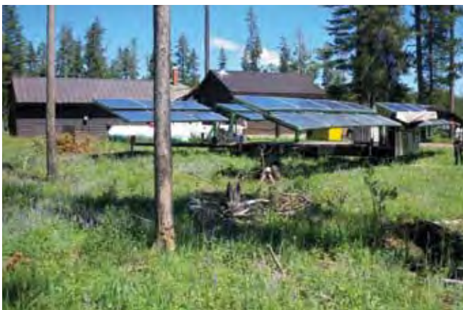
This portable photovoltaic system at Bechler provides power during the summer season, meeting 90 percent of the site's electrical needs.
