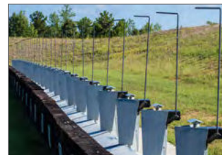
Mounted upright to a concrete pad (w/ballistic shield)
