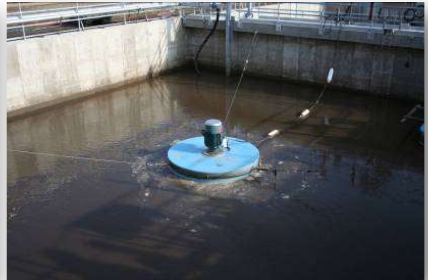
Anoxic Mixing (Denitrification and Power Savings)
