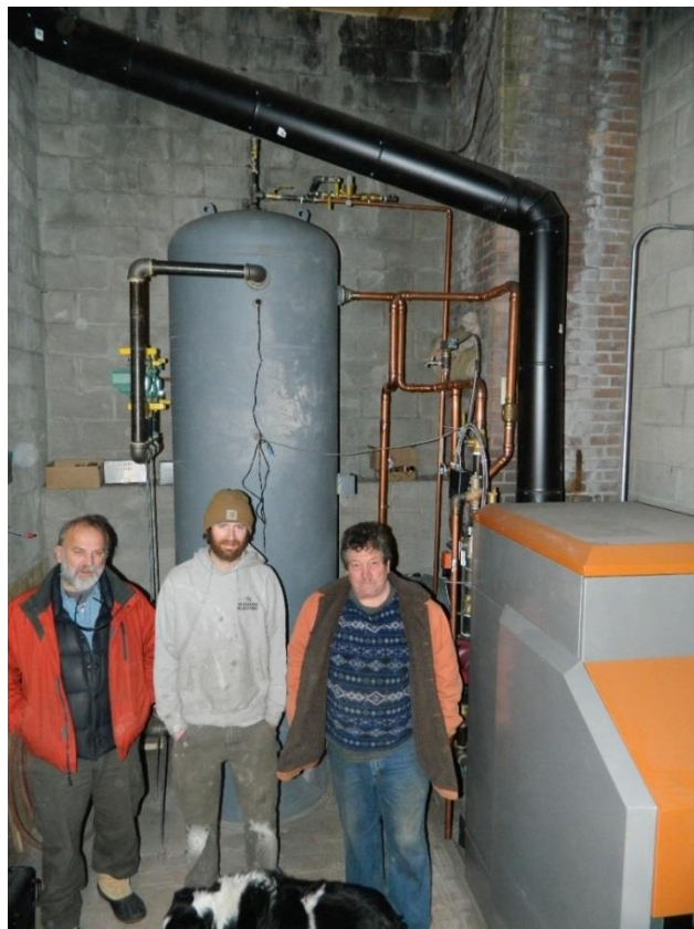
Figure 2 - Near completion of the install. Left to Right: Rob Steingress (VFFC Treasurer), Bill Kretzer (12 Gauge Electric), and Greg Cox (VFFC President).
