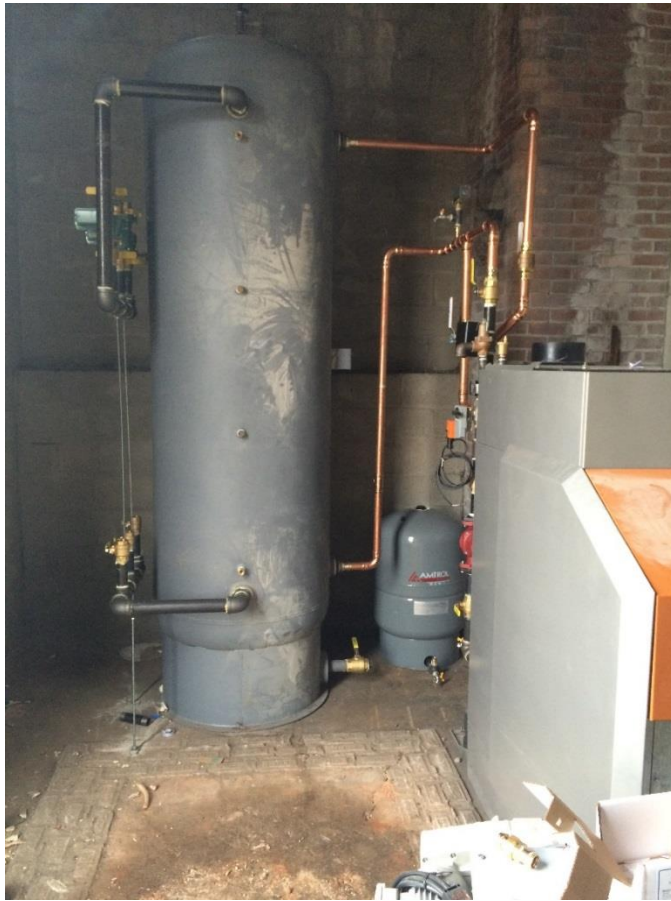
Figure 10 - The 600 gallon buffer tank (left) allows heat to be transferred to the building as soon as it is needed while the boiler (right) fires up and gets to temperature. The primary circulation loop is between the boiler and the tank. The circulators for heat distribution to the building are the green items in the upper left. This picture was taken prior to insulation of the tank and piping.
