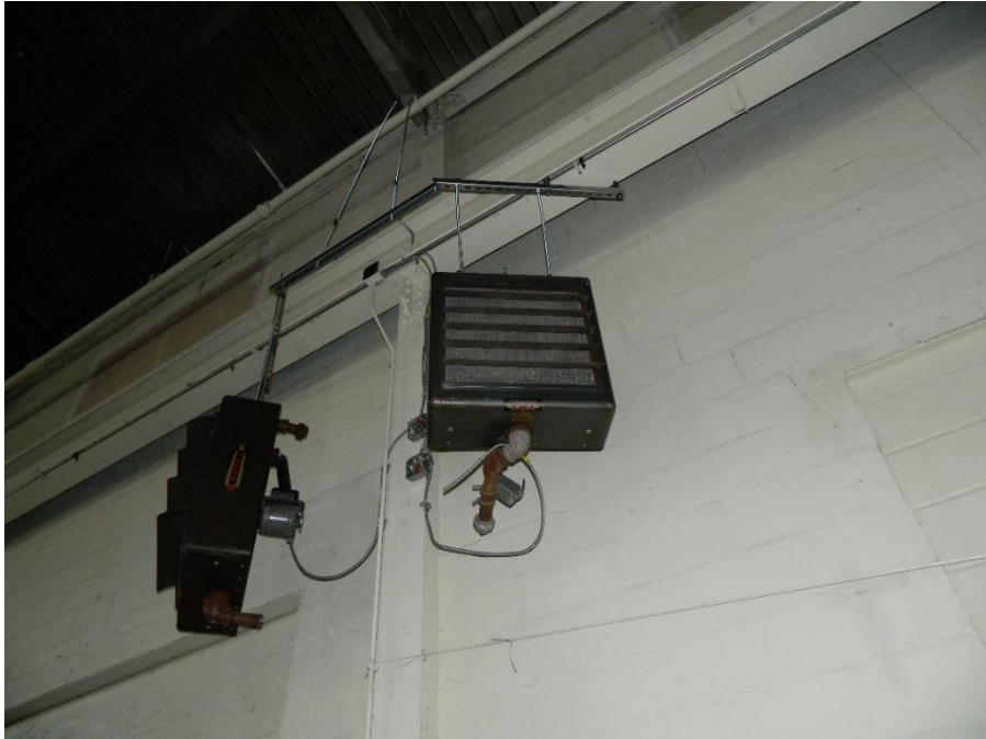
Figure 13 - Two of the cast iron hydronic / steam unit heaters salvaged from the site and reused for this new heating system find a new home above Farmer's Hall.
