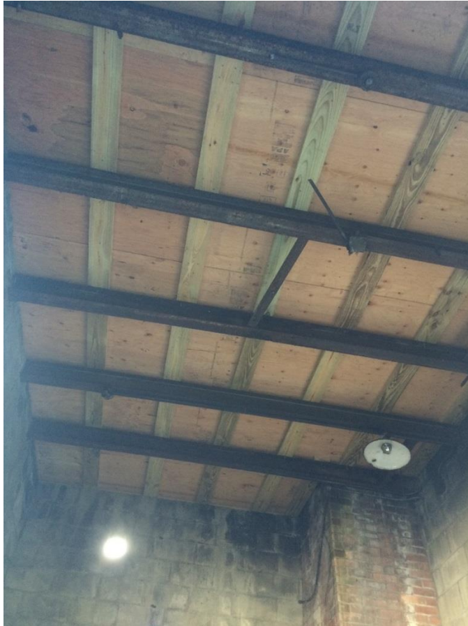
Figure 6 - The ceiling of the renovated boiler room showing new roof decking on top of the existing steel structure.
