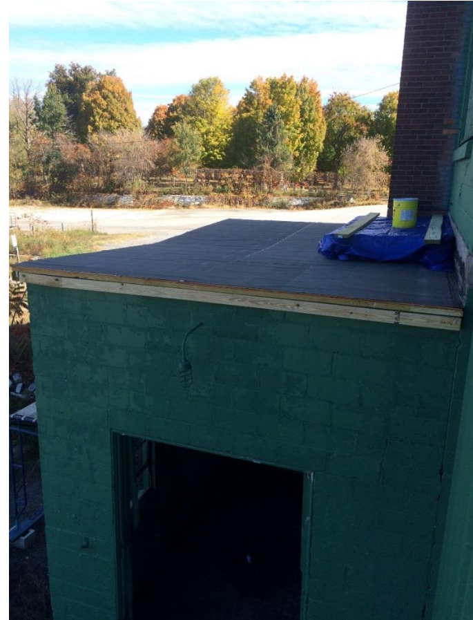
Figure 7 - The top of the boiler room showing the new roof. The dip at mid-span is intentional to allow for flow of stormwater off of the roof.
