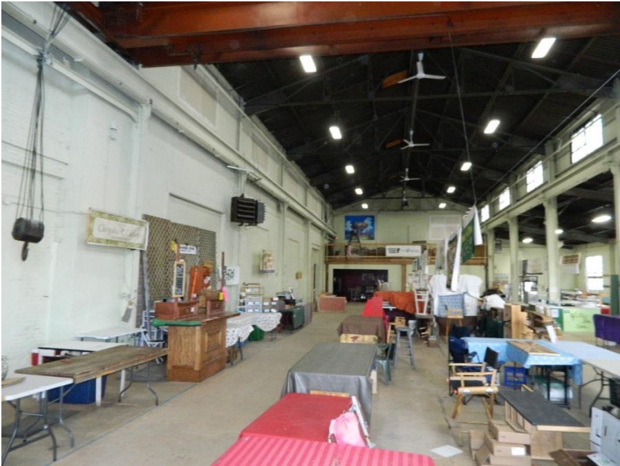
Figure 15 - Farmer's Hall the VFFC with two of the hydronic unit heaters in place (left).
