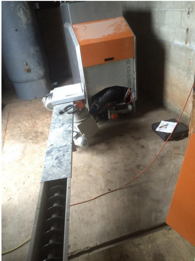
Figure 8 - The boiler, tank, primary auger and combustion feed auger set in place as a "dry fit" prior to final plumbing to allow for locating the boiler in the room.
