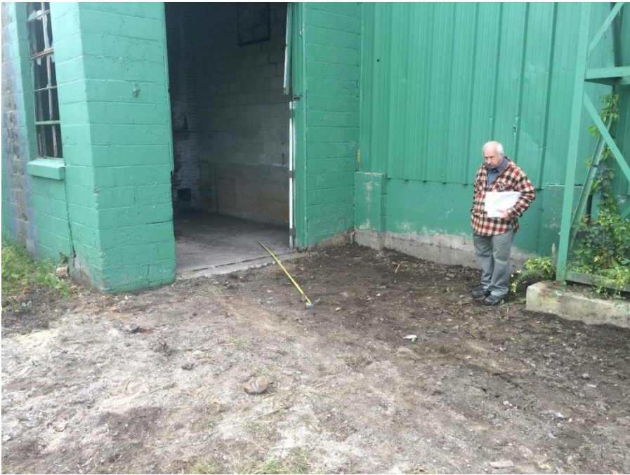
Figure 3 - Laying out the fuel bin. The measuring tape is set to 10 ft of length to illustrate the rough location of the primary feed auger. Charlie Brown (Smalley Mechanical) provided engineering support of the project.
