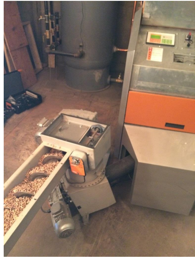
Figure 11 - The primary feed auger filled with wood pellets during normal operation of the boiler at VFFC in late Winter 2016.
