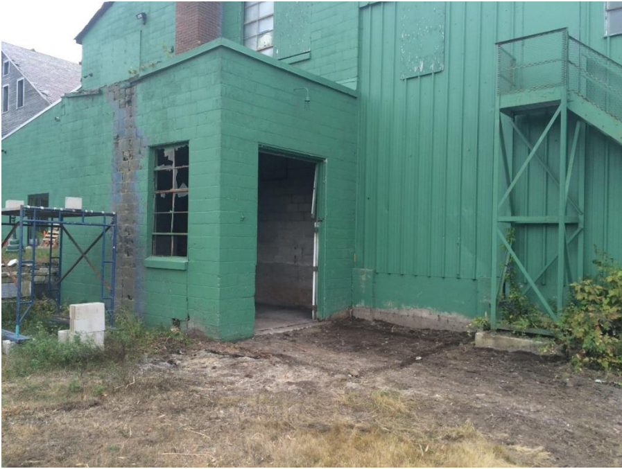
Figure 4 - The exterior of the boiler room after initial cleanup, but prior to new doorway (in place of window) and prior to the construction of the fuel bin (off of the large opening in the center of the view). The bin foot print is outlined in the dirt.
