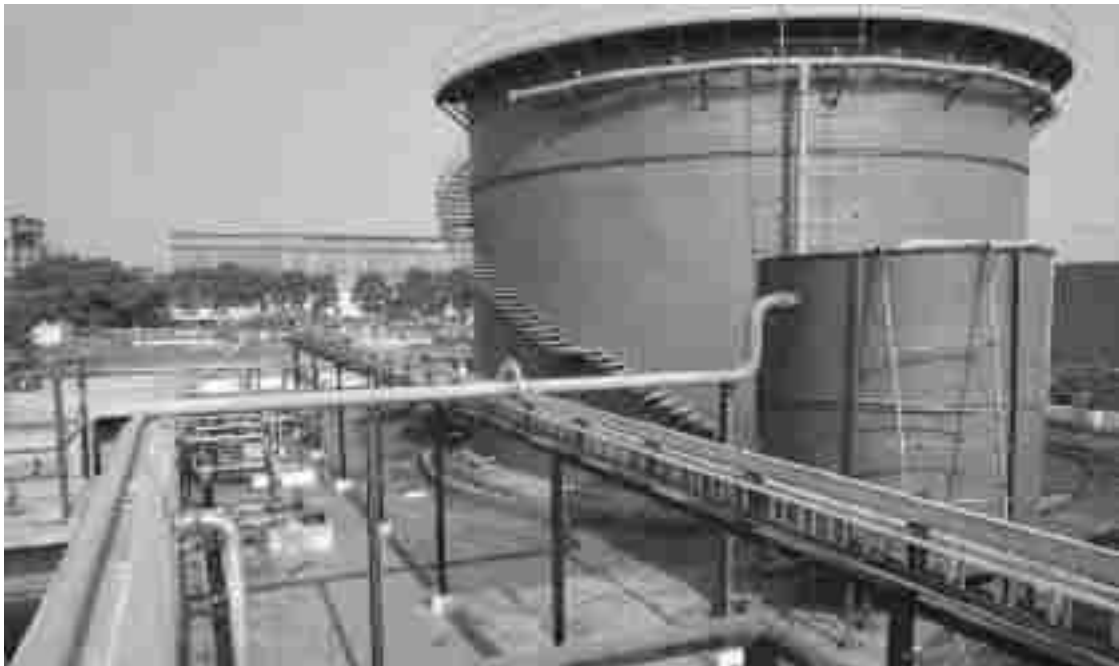
Pic :- 6 CPU (UASBR)
