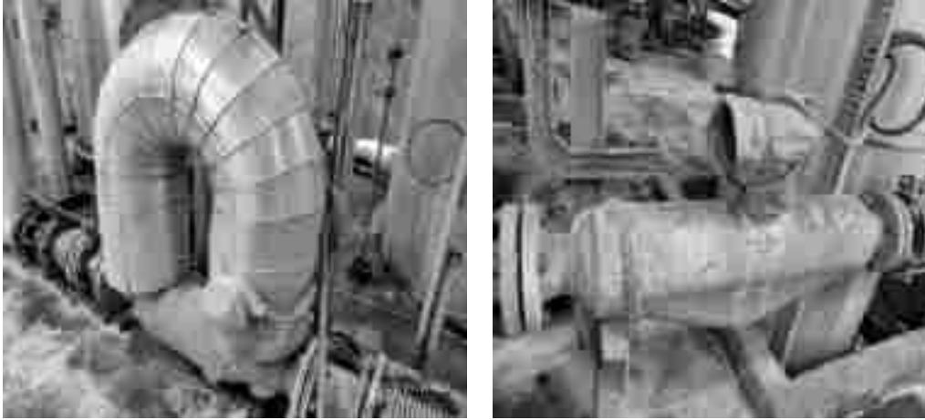
Pic-7 Mass Flow Meter Inlet/Outlet Of MEE Plant
