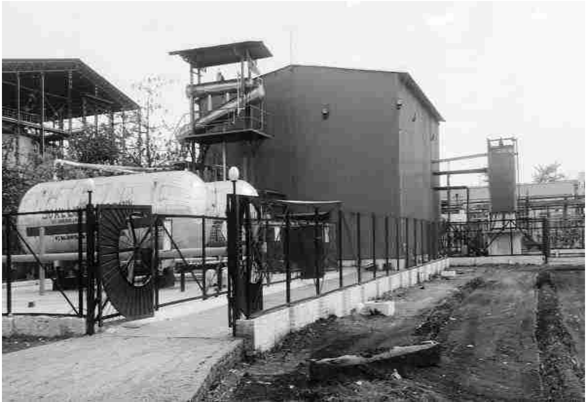
Pic-15 Co 2 Plant
