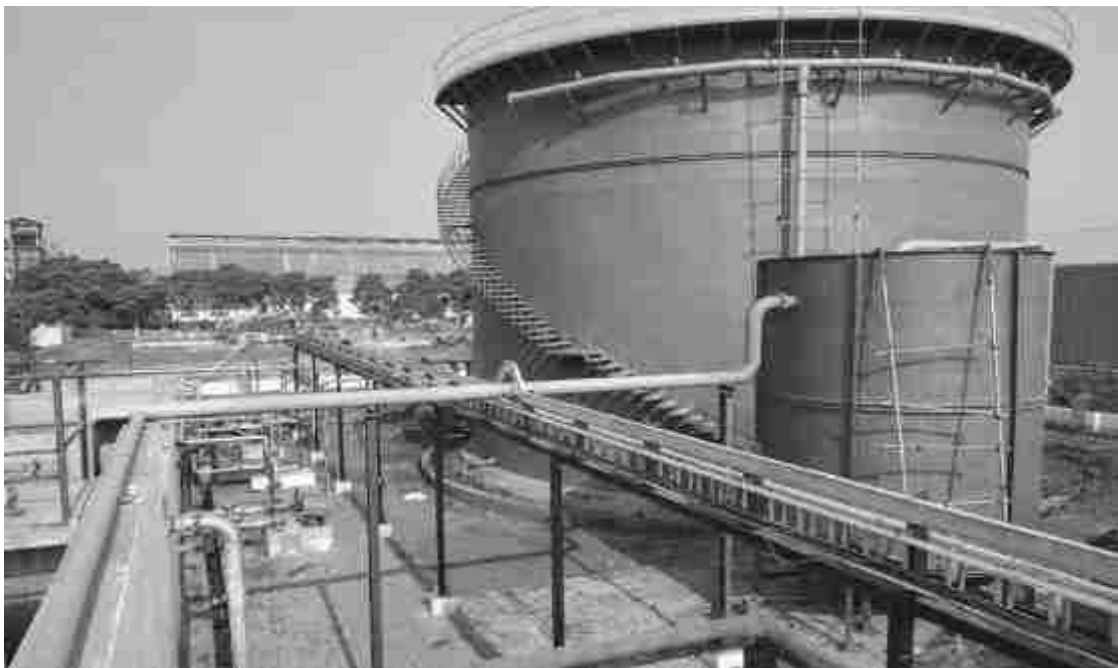
Pic :- 4 CPU (UASBR)
