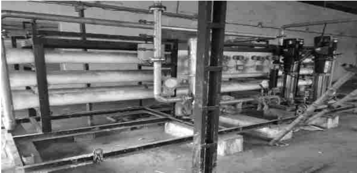
Pic :-5 RO Plant
