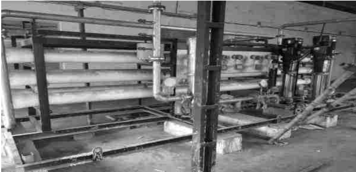
Pic :-5 RO Plant
