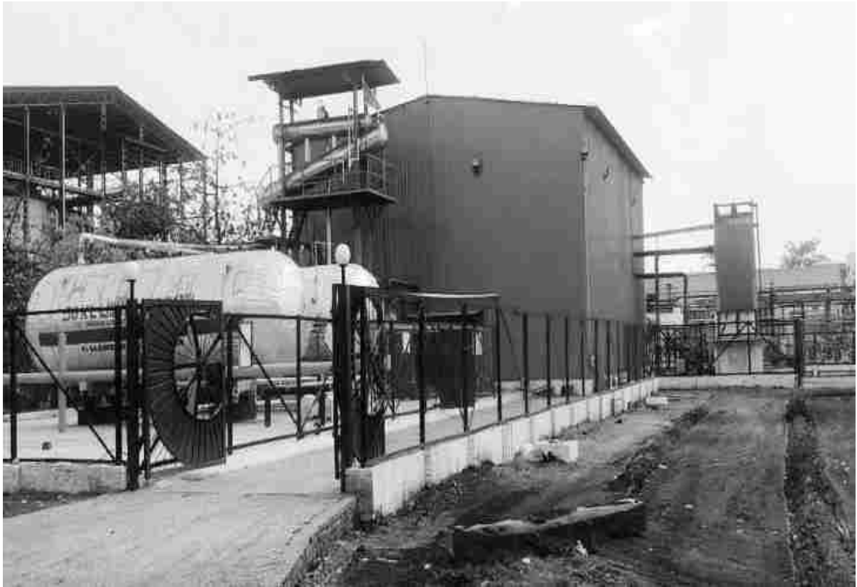
Pic-15 Co 2 Plant
