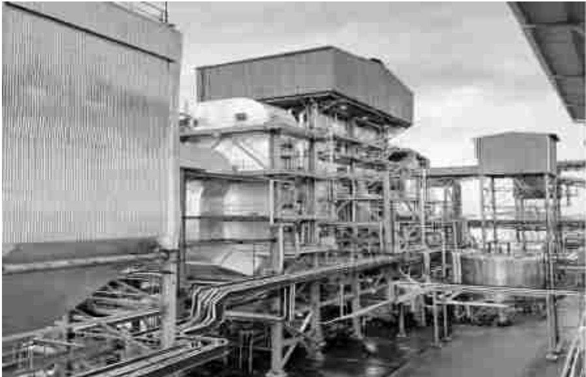
Pic :- 3 Slop fired Boiler alongwith ESP (Incineration Boiler)
