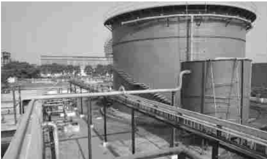
Pic :- 4 CPU (UASBR)
