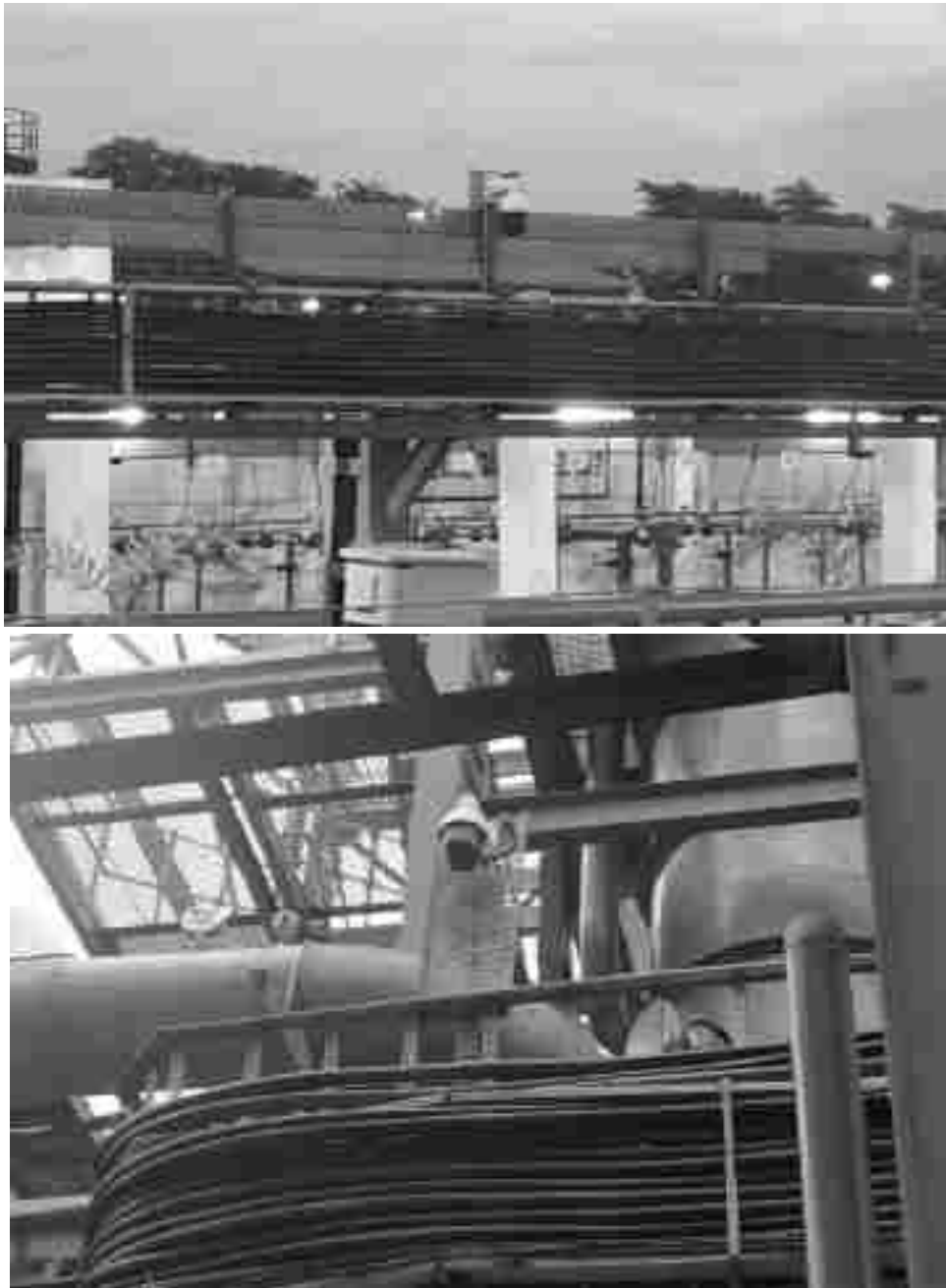
Pic- Two Nos. Of Web Camera at Spent wash Storage Lagoon & MEE/Incineration Area
