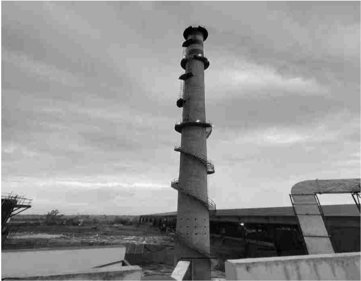
Pic :- 1 RCC Stack (Height -80mtr) alongwith Online Dust Monitoring System
