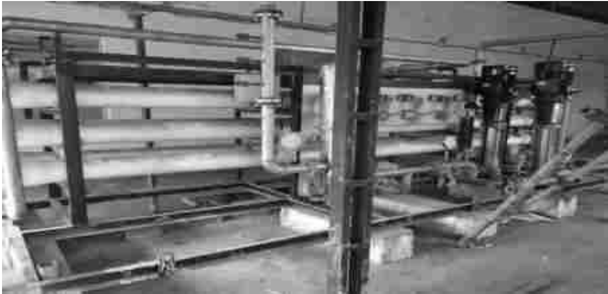
Pic :-7 RO Plant
