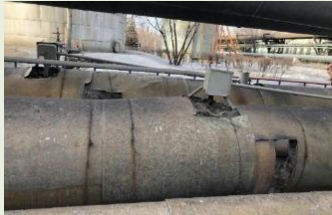
6. Observed insulation damage
