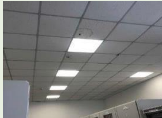
2. Stain due to water leakage
