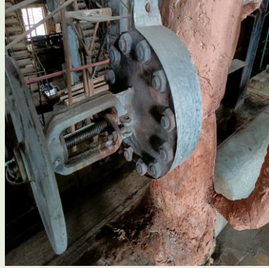
2. Steam line insulation damaged
