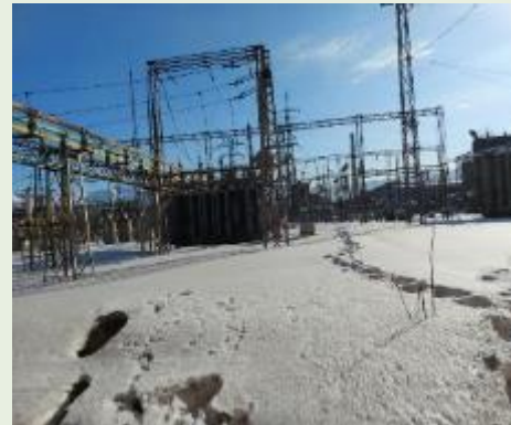
10. Switchyard: Well maintained and colour coded
