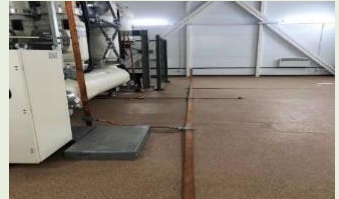
3. Bare earthing copper strip
