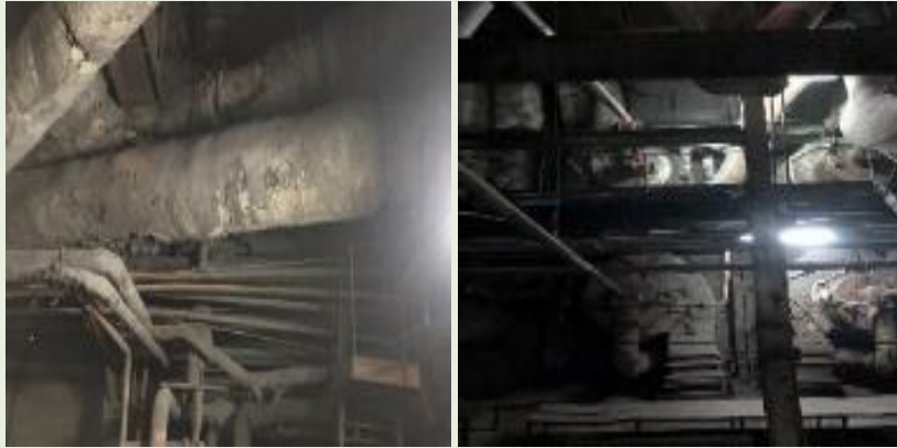
4. Suspended coal dust and damaged insulation
