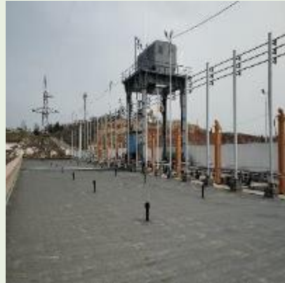
8. Crane for maintenance of sluice gates
