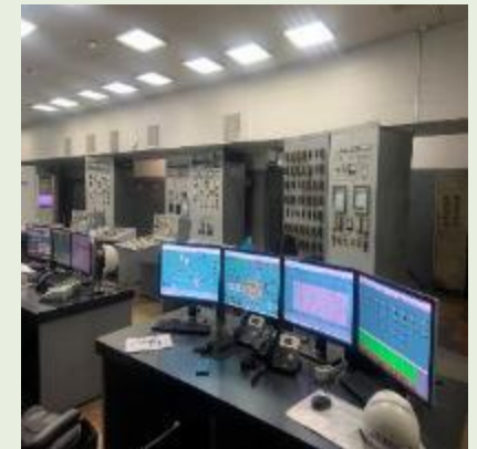
6. Control room: manual knob operation
