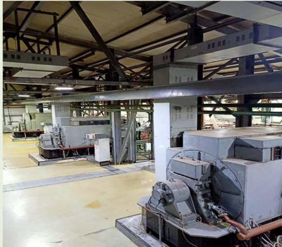
1. Gas turbine generator hall
