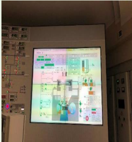
1. No vibration parameter in DCS screen
