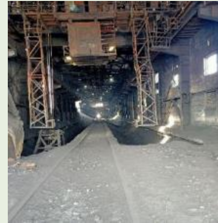
7. Coal unloading station
