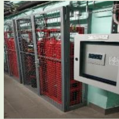
2. Fire extinguishing system in TG floor
