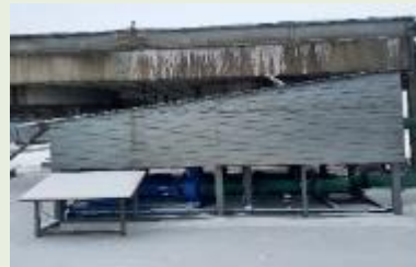
2. Oil cooling system
