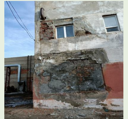
4. Damage to building structures
