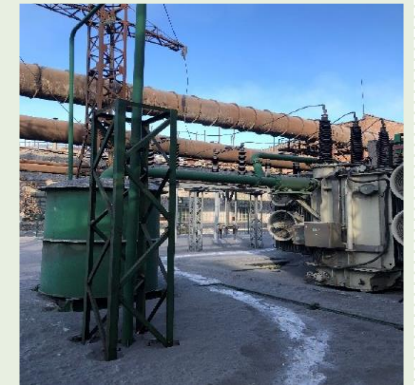
4. Fire fighting system
