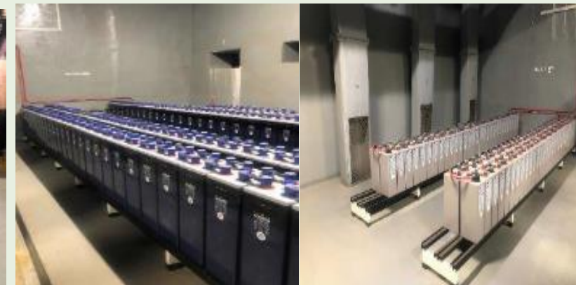
3. DC battery bank room was clean and well maintained
