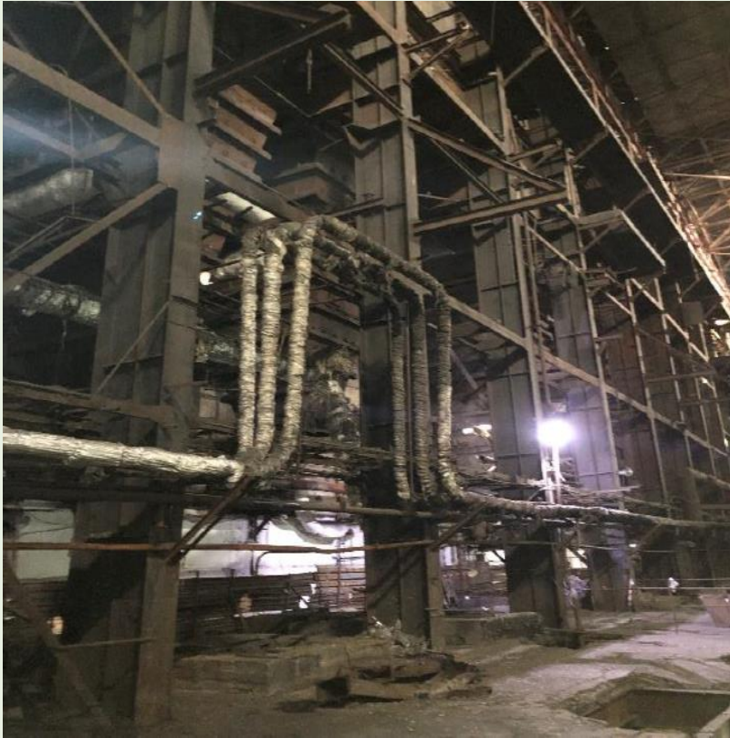
1. Poor Insulation of piping structures
