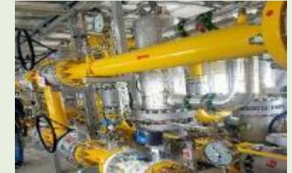
4. Natural gas filtering system
