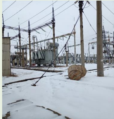
2. Switchyard and main transformers
