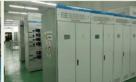
3. Switchgear and auxiliary transformers
