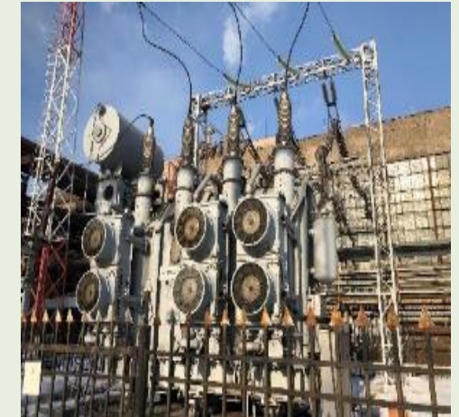
6. Transformers: lack enough fire fighting system
