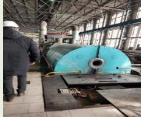
7. STG hall : Flooring plates are removed - no caution sign or fencing
