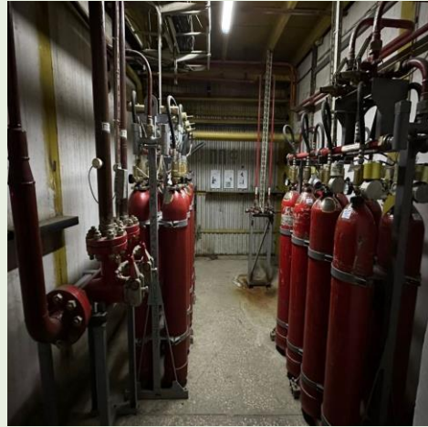
2. Fire suppression system
