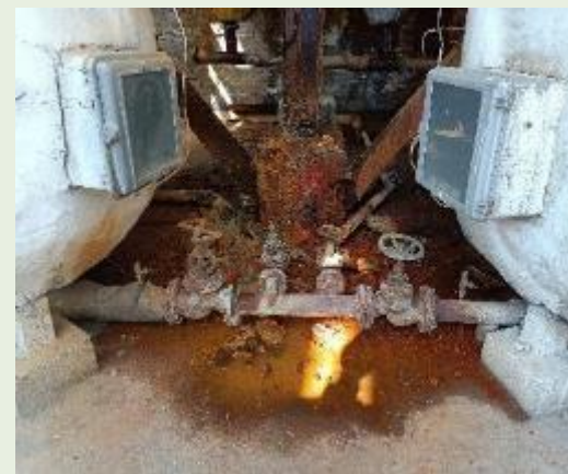
3. Boiler flash tan leakage
