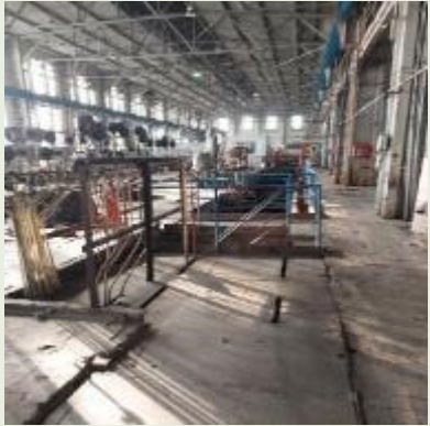
1. Damaged and unlevelled flooring in STG hall
