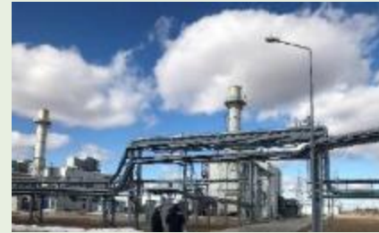
3. Piping and clear flue gas from chimney
