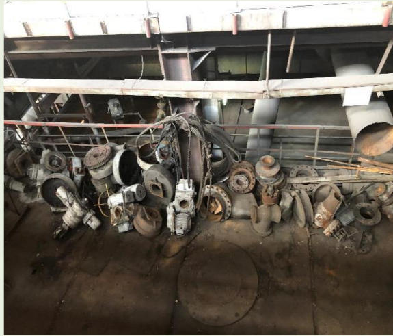
1. Poor equipment maintenance
