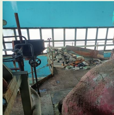
8. Debris accumulated on turbine floor
