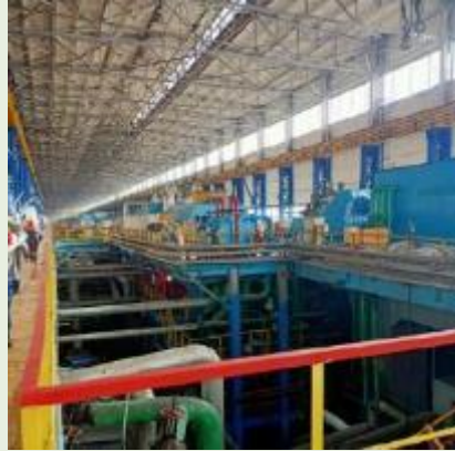
2. Turbine generator hall
