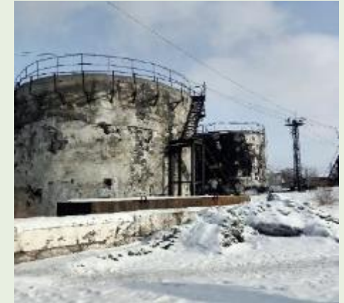
4. Storage tank damage
