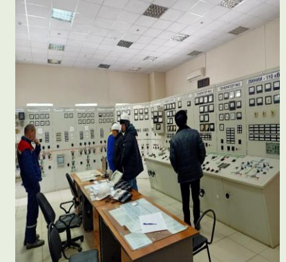
5. Control room - manual knob operations
