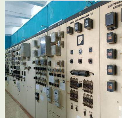
9. Mechanical relay panel
