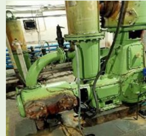
7. Rusting and damage in air compressor
