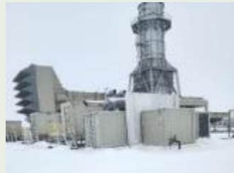
1. Gas turbine and generator
