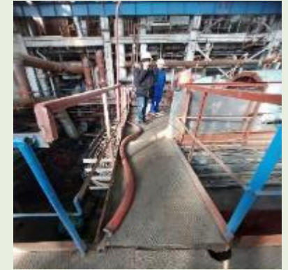
5. STG hall: Inadequate maintenance of wires, pathways, and fire hydrant system
