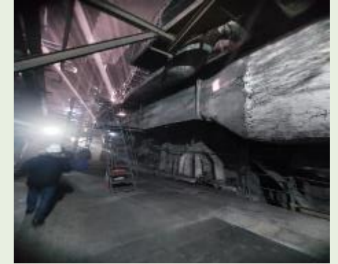
8. Boiler floor area: Combustion air duct refractory damaged
