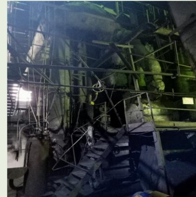
3. Poor pipe insulation
