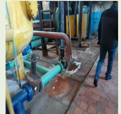
8. Water and chemical leakage in water treatment plant
