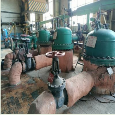
1. Hot water heaters - insulation damaged
