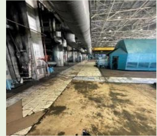
3. Damaged flooring risk of trip and fall accidents
