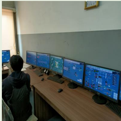
6. New boiler control room with DCS
