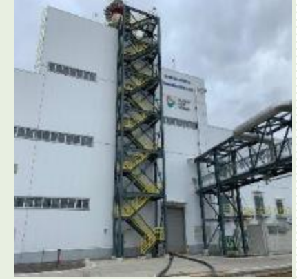
5. Plant outside - well maintained and regulated
