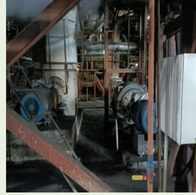
3. Coal dust near new boiler units
