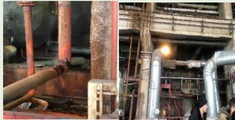
2. Leakages and spills from pipe structures
