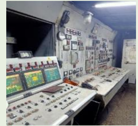
8. Boiler/turbine control room
