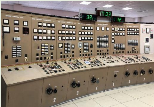
4. Power plant control room
