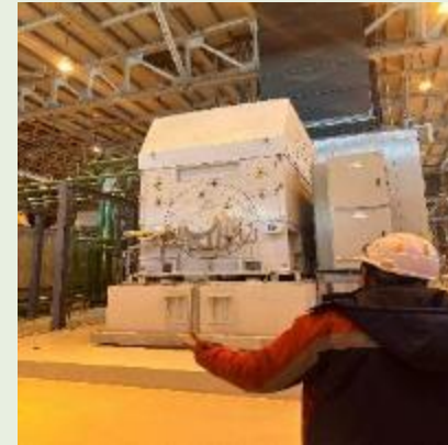
4. Turbine hall: clean and equipment are new
