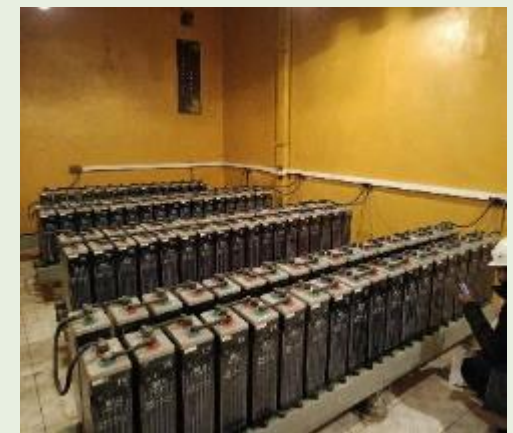
4. Battery bank - no safety sensors
