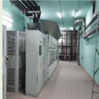
5. Switchgear for auxiliary transformers
