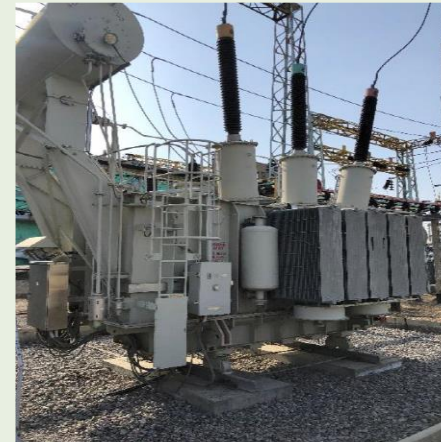
4. No fire wall for transformers/ CO 2 flooding system
