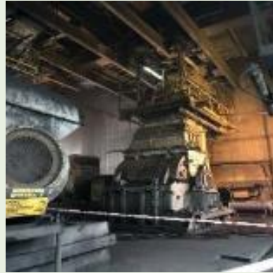
2. Cables and water spillage around crusher
