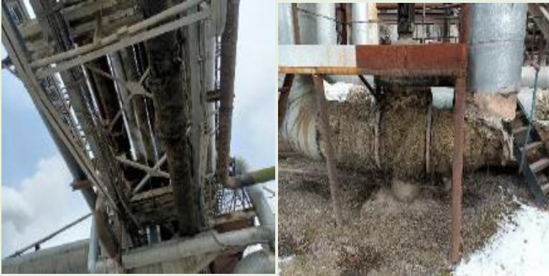
4. Improper/No insulation to the piping and equipment
