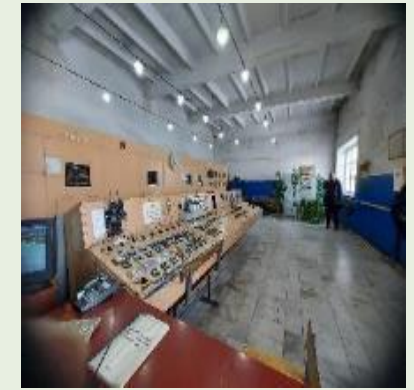
4. Control room had manual knob operations
