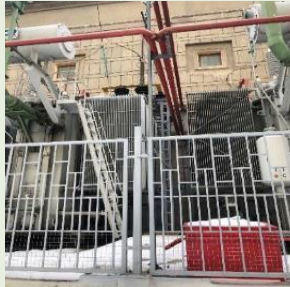
2. No fire barrier wall
