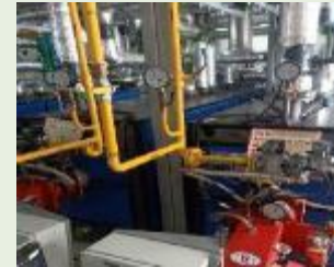
3. Natural gas heating system
