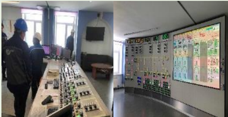
1. Control room was well equipped with DCS but had manual knob operations
