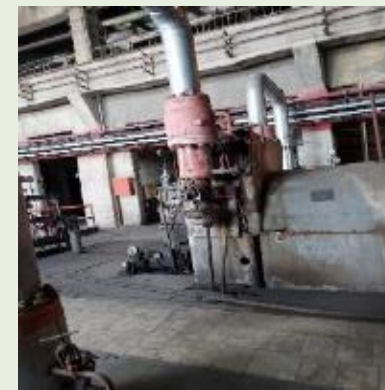
3. Rusting of equipment
