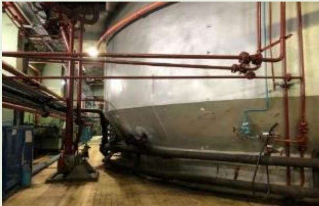
1. Low and unsupported piping
