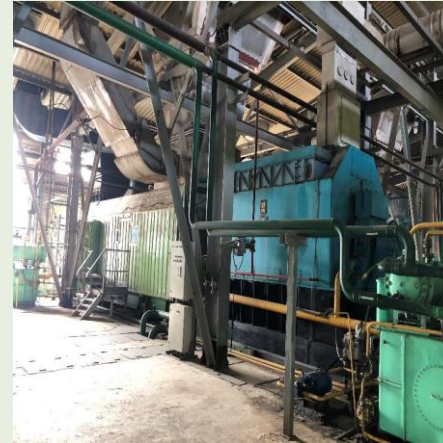
2. Turbine generator unit
