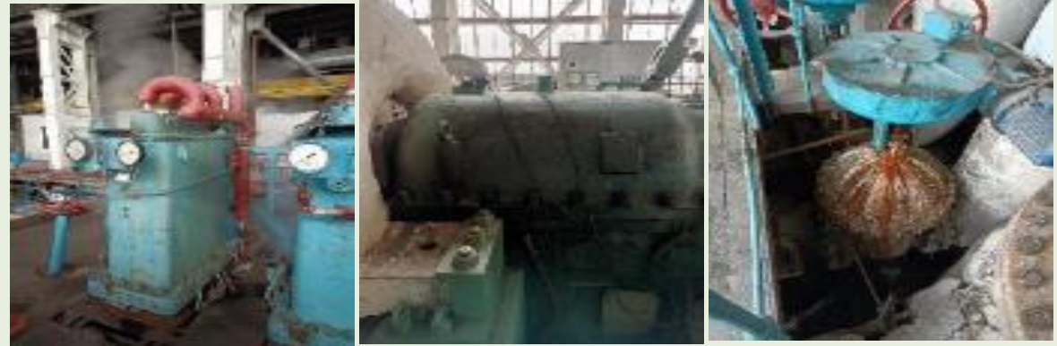
6. Steam/Water leakage observed in the plant
