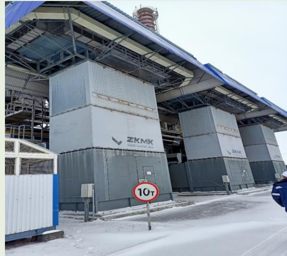
2. Air filter house
