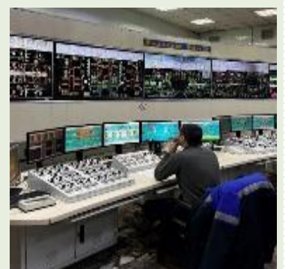
4. Control rooms for units with manual knob operations
