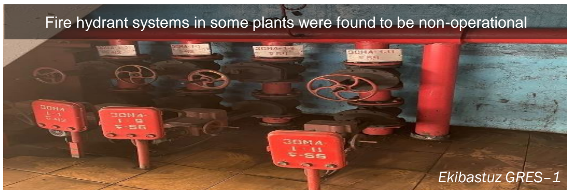
Unpreparedness for fire hazards
