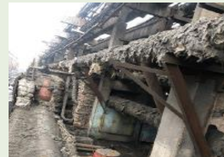
7. Insulation damage on outdoor pipes
