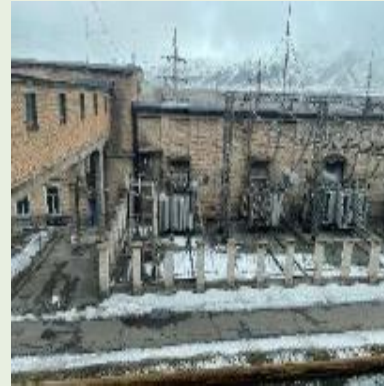
5. No fire barrier wall between each transformer 2
