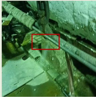
2. Steam leakage in the pipes
