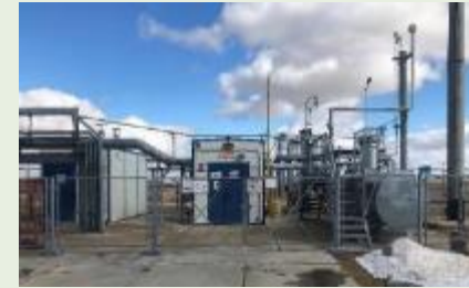
4. Gas filtering and pressurizing station
