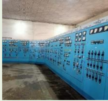
2. Electrical control room
