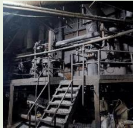
6. Coal dust in boiler floor
