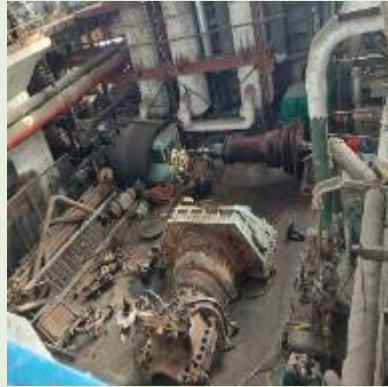
2. Maintenance bay: Dust accumulation and no fire extinguishers
