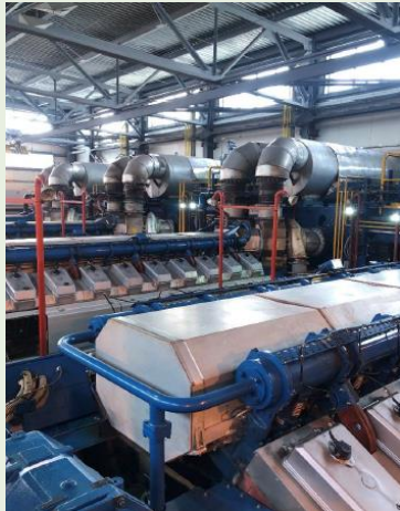
1. Turbine generator unit
