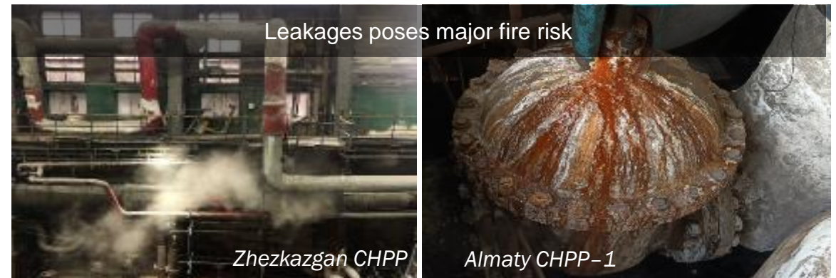
Steam, water, oil, oil fume leakages
