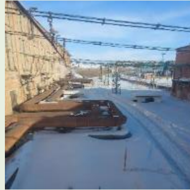
3. Steam pipelines: External surface rusted
