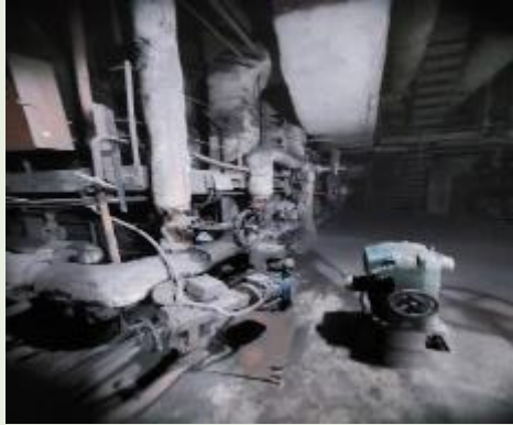
6. Boiler floor area: Grease and coal dust accumulation on equipment
