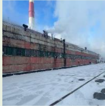
2. Old and damaged walls in the plant
