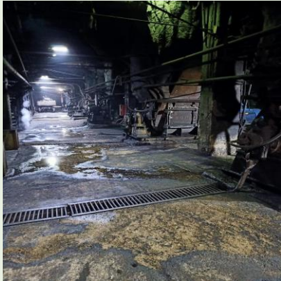
1. Water leakage from the boilers
