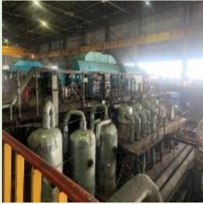
1. Turbine room: coal dust accumulation over equipment
