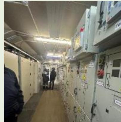
3. Controls and monitors
