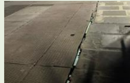
3. Trip and fall hazards
