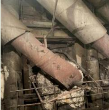
1. Damage on civil structures
