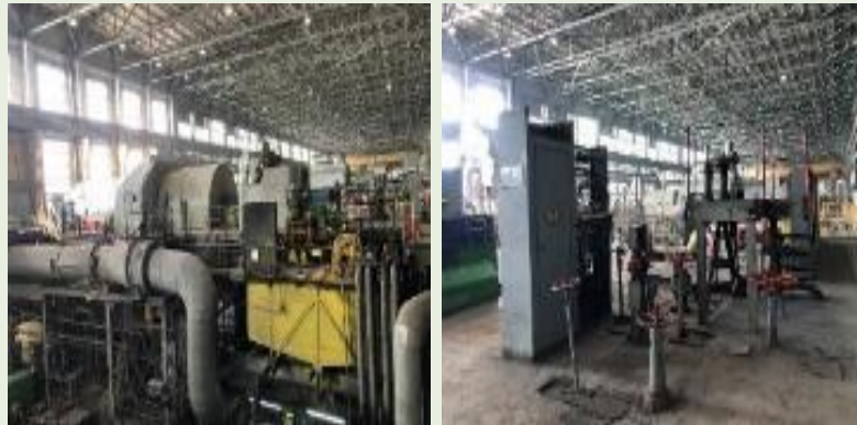
7. No proper tagging, oil leakage, steam leakage, no fire fighting system
