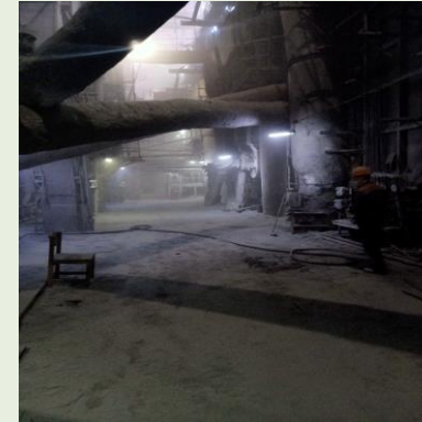
3. Poor maintenance of the boiler room 1
