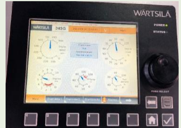
4. Generator human machine interface (HMI)
