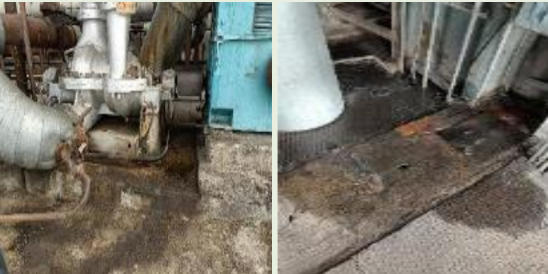
5. Oil leakage observed in the plant
