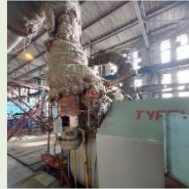
4. Governing valves: Damaged insulation and glass wools
