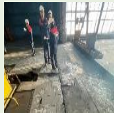
2. Cracks on floors and structures, and corrosion
