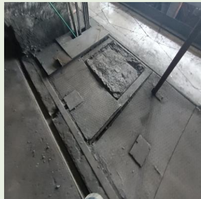
4. Cover plates not aligned properly
