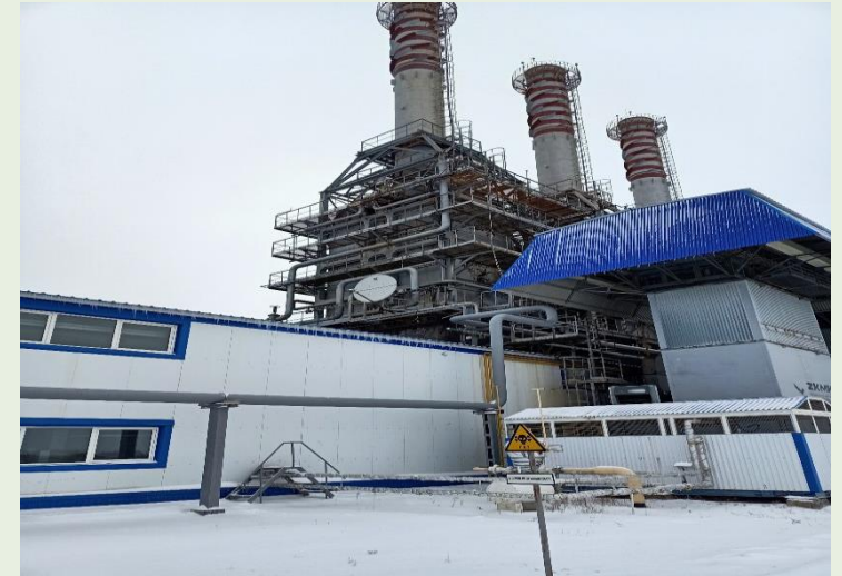
3. Boiler 1 - currently out of service
