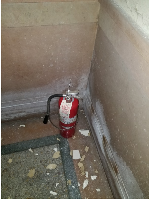
Portable Fire Extinguisher
