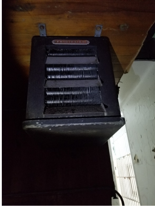
Ceiling Mounted Air Conditioner
