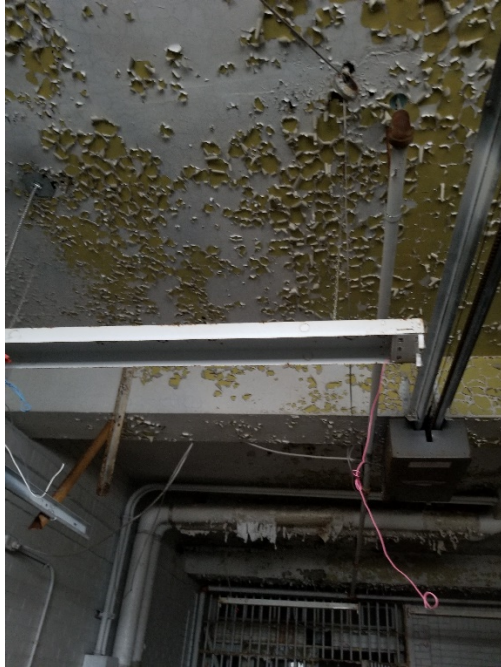
Peeling Paint Basement Ceiling
