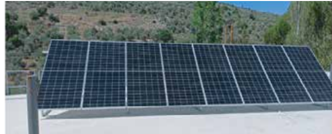
Figure 2: Solar panels installed within the Hasbaya Living Lab
