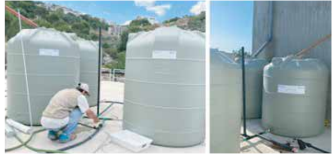
Figure 1: Water harvesting units installed within the chosen sites
