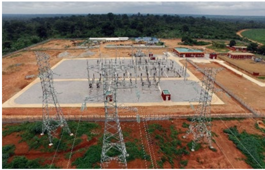
Transmission lines and infrastructure in Côte d'Ivoire.
