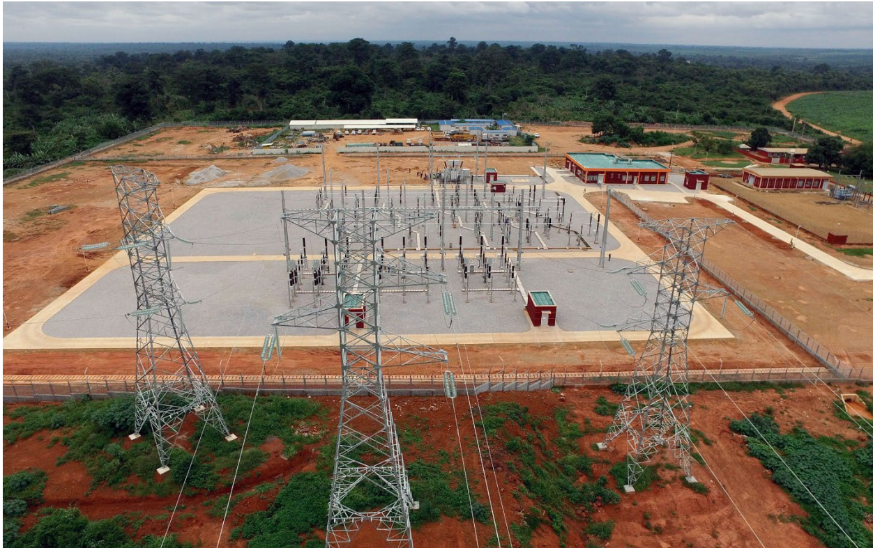
Figure 5: Photo of HV Transmission Switching Station in Cote d'Ivoire. Photo Credit: @PAWAEP
