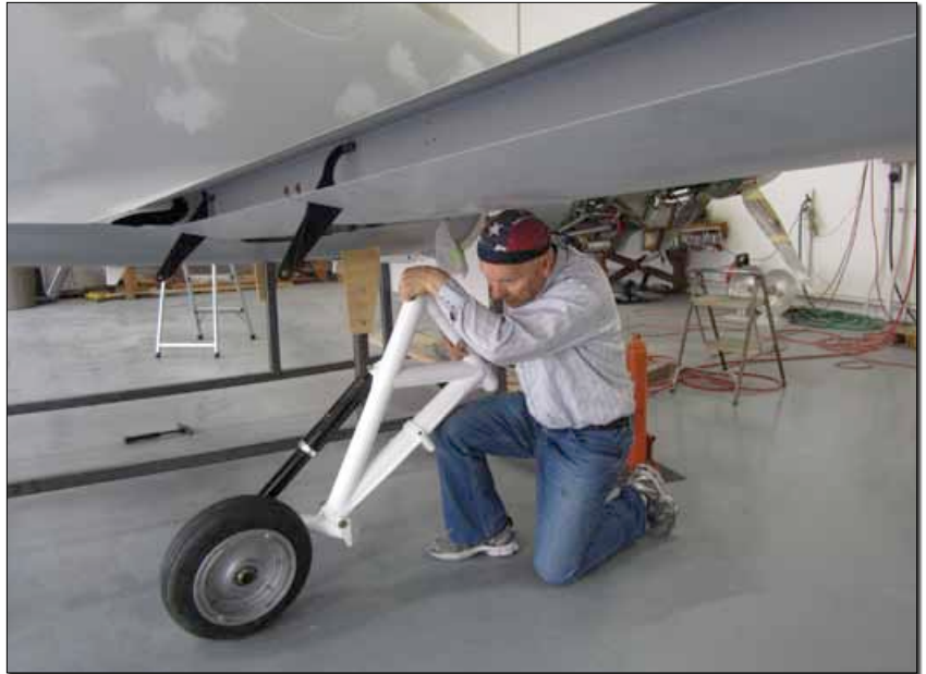
Wendell installs the new, beefed-up steel landing gear provided by Lancair after the original aluminum gear legs proved to be a bit too fragile. Lancair has been very good about providing these upgrades free to early kit builders.
