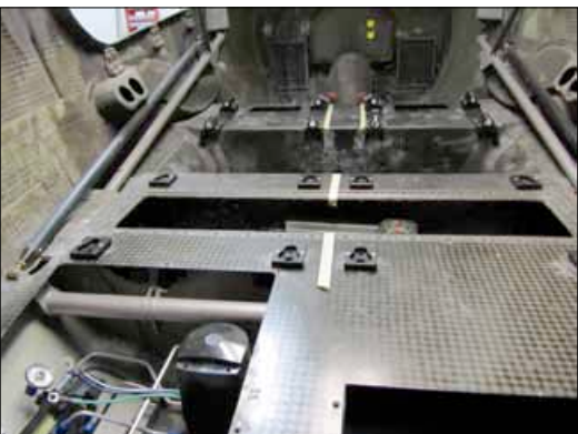
There is a lot happening under the cabin floor of the Evolution. Several access panels cover up the systems underneath. The hydraulic pump for the landing gear can be seen on the lower left.
