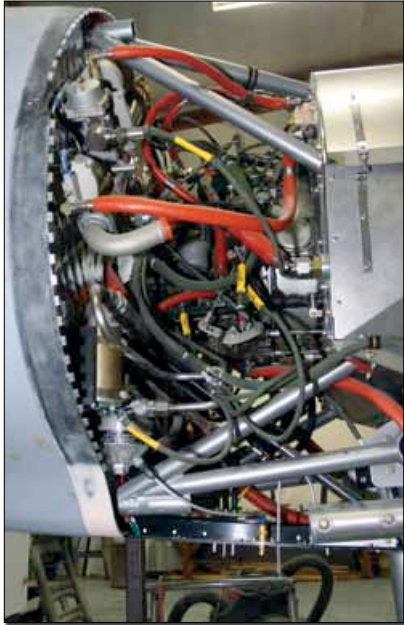
The space between the engine and the firewall is a busy place in the Evolution engine compartment. In this photo the flow pack and gascolator stand out. Beyond that it looks like a big bowl of spaghetti, but the Solesbees know where everything goes, or so we hope.
