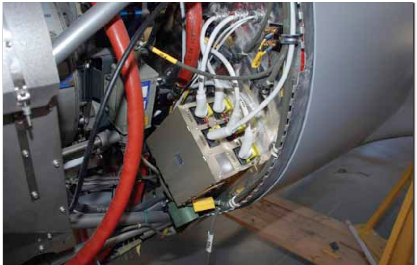
Big power needs big wires. Those king-sized wire crimpers come in handy when putting ends on the #1 and #2 AWG wires that run from the batteries and the starter/generator. The power control unit handles all the power switching, routing and regulating duties for the Evolution. In most homebuilt airplanes, each of these chores is handled by separate components.
