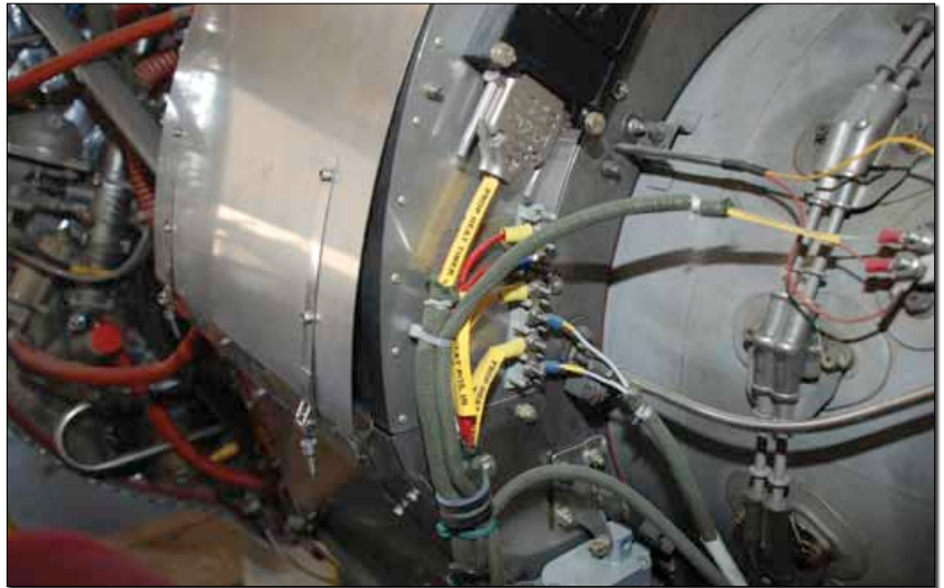
Pre-wired electrical harnesses make wiring easy for the Evolution builder. The clear labeling on these harnesses speeds up the work and ensures that wires go where they are supposed to.
