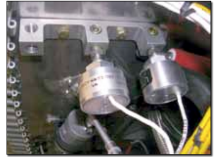
Mounting these sensors directly to the firewall ensures good ground contact.
