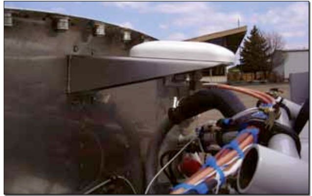
More secured coax cables bundled with other wires along an engine mount tube.
