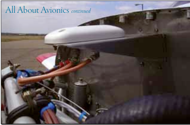
The coax cables secured to this engine mount tube are routed through cushion clamps and wire ties.
