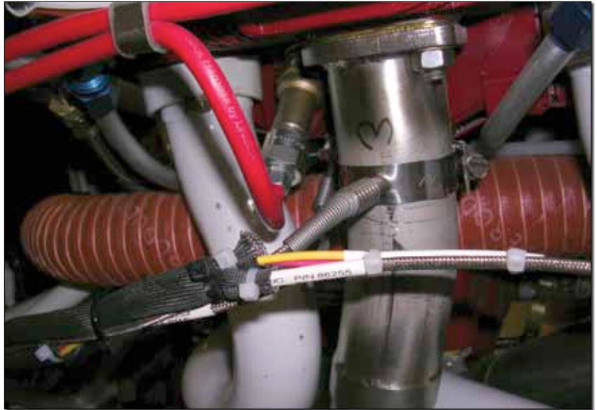
Devices such as exhaust gas temperature (EGT) probes need to be adequately mounted, secured and protected.
