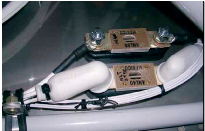
Protective boots over heavy wire terminals can be beneficial.
