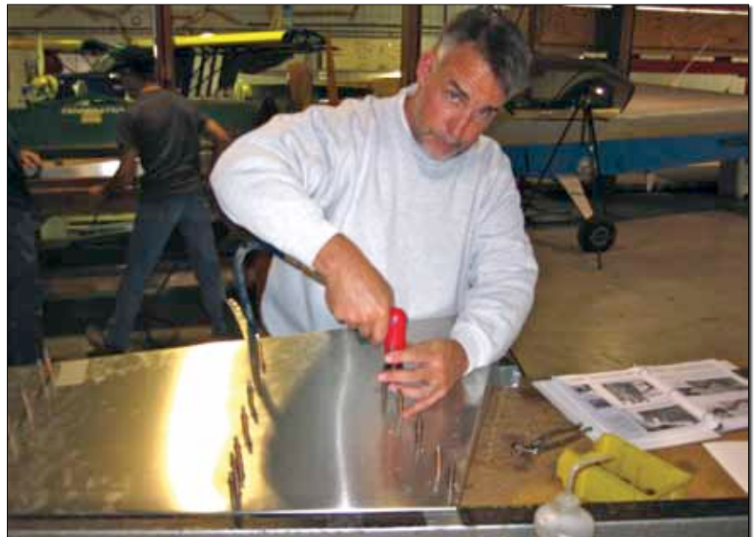
When you don't have a project of your own, borrow one. The author at the Zenith Aircraft build-a-tail day last year, trying to remember how a pneumatic drill works.
