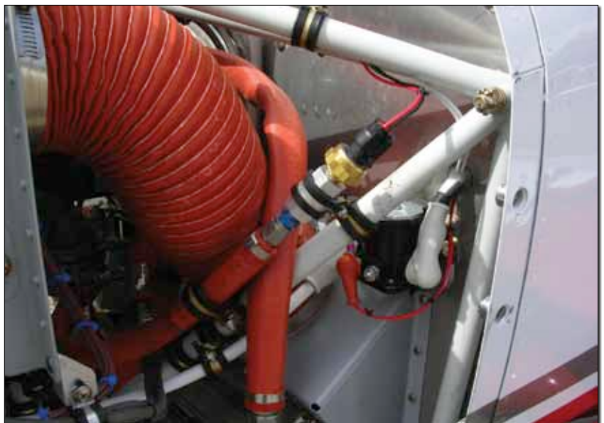
This clean installation shows use of protective boots, cushion clamps and clean wire routing.
