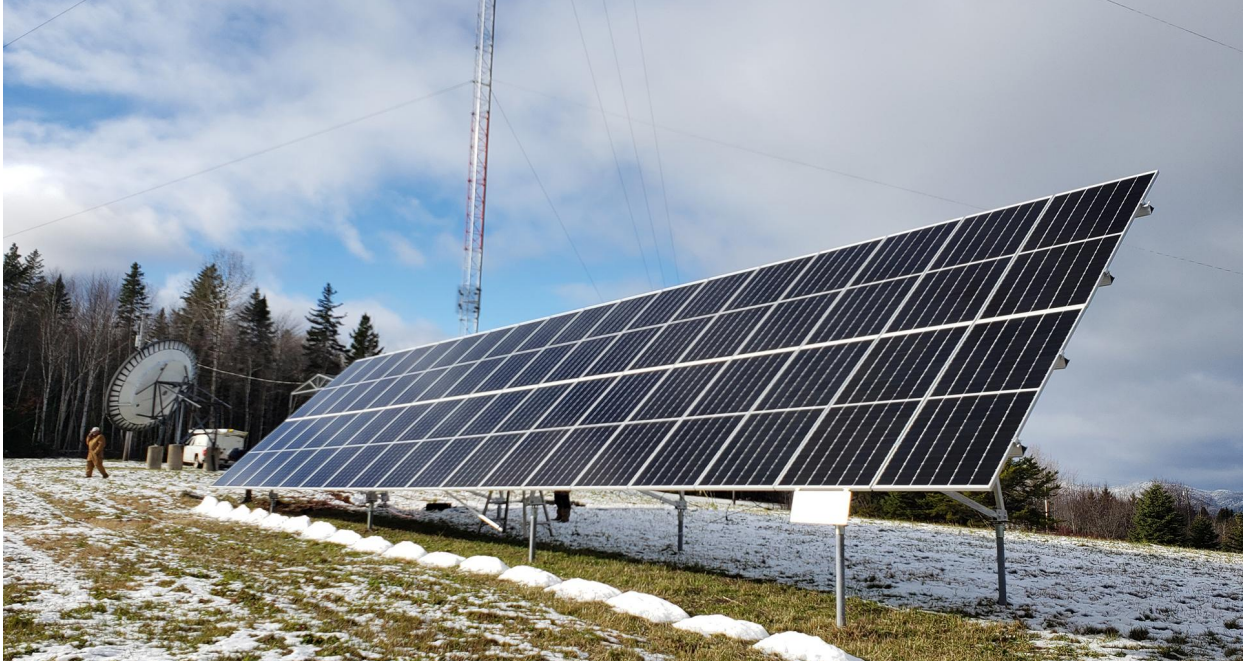
The solar panel located in Pointe La Nim, New Brunswick.
