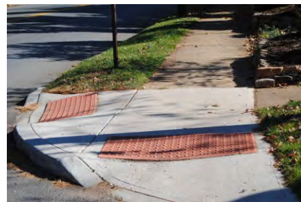
CSO work provided the opportunity to install curb ramps increasing pedestrian movement.
