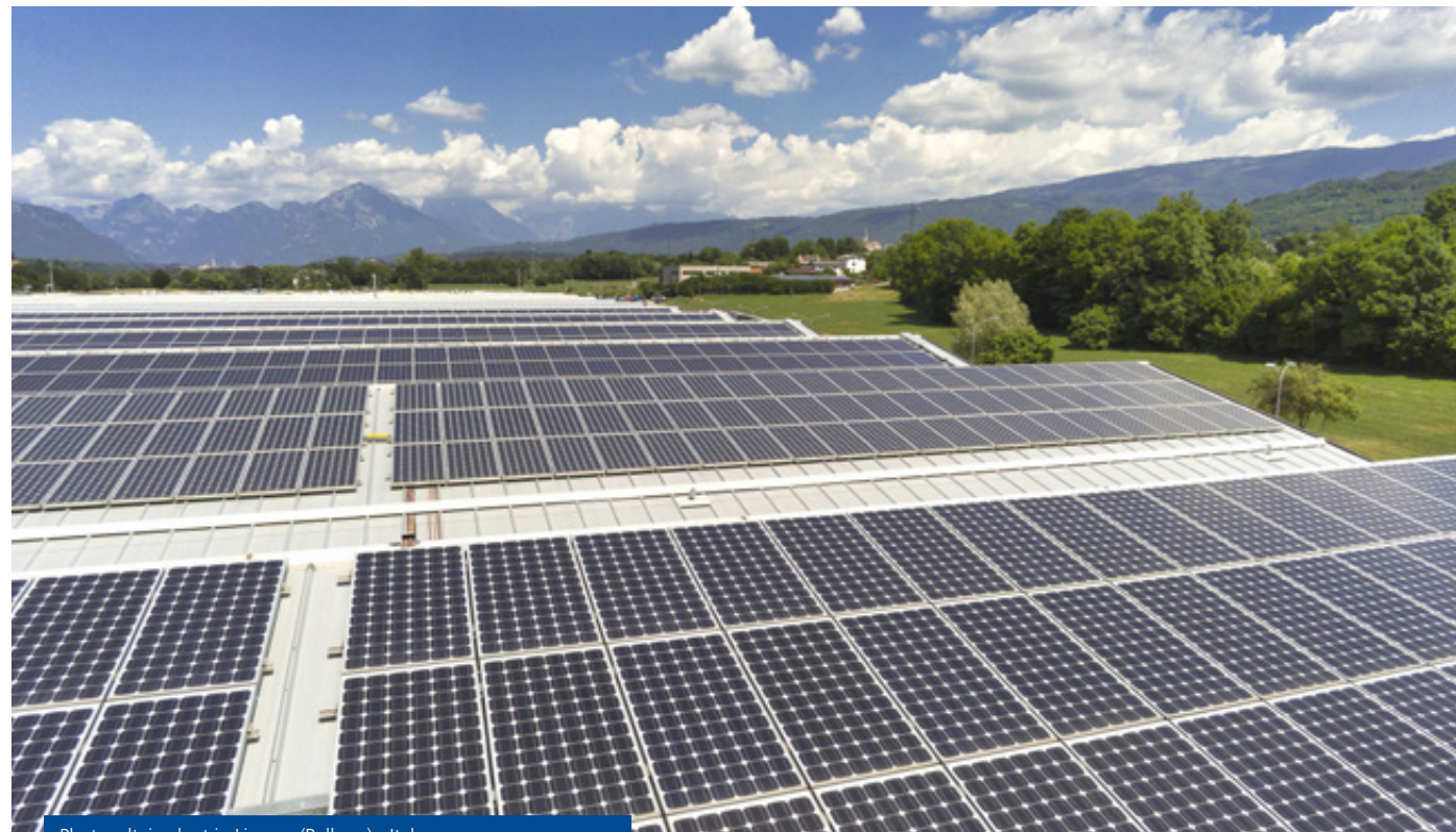
Photovoltaic plant in Limana (Belluno) - Italy
