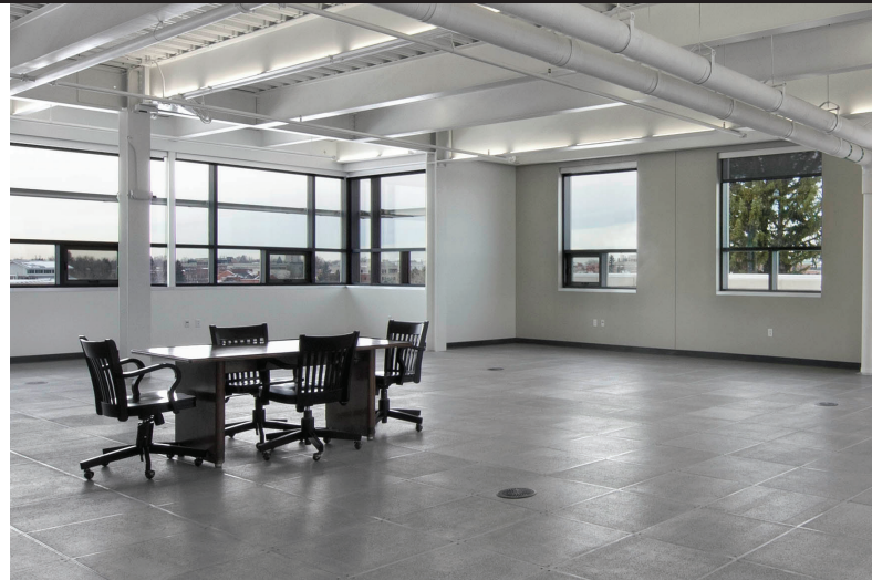
Fresh air moving under the floor is conditioned prior to entering the room through the vents shown. LED light bars are mounted to overhead beams.
