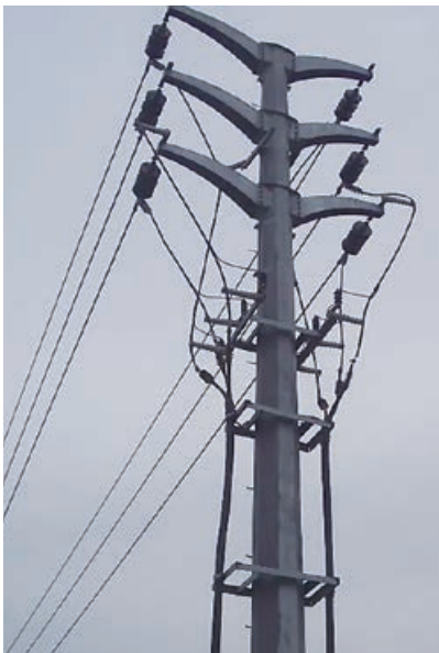
Steel Monopole Tower (NTSMT-003)
