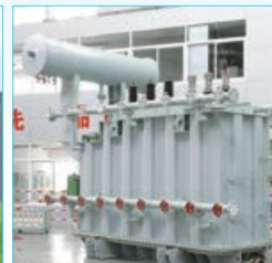
Power Transformer (SFSZ10-50MVA 110KV)
