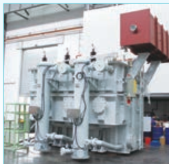
60 mva Eaf Transformer (SSPT-60 MVA-33KV)
