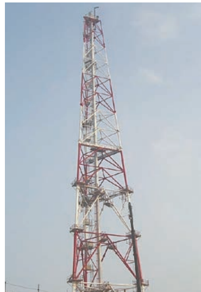
Steel Broadcast Mast (NTSBM-009)
