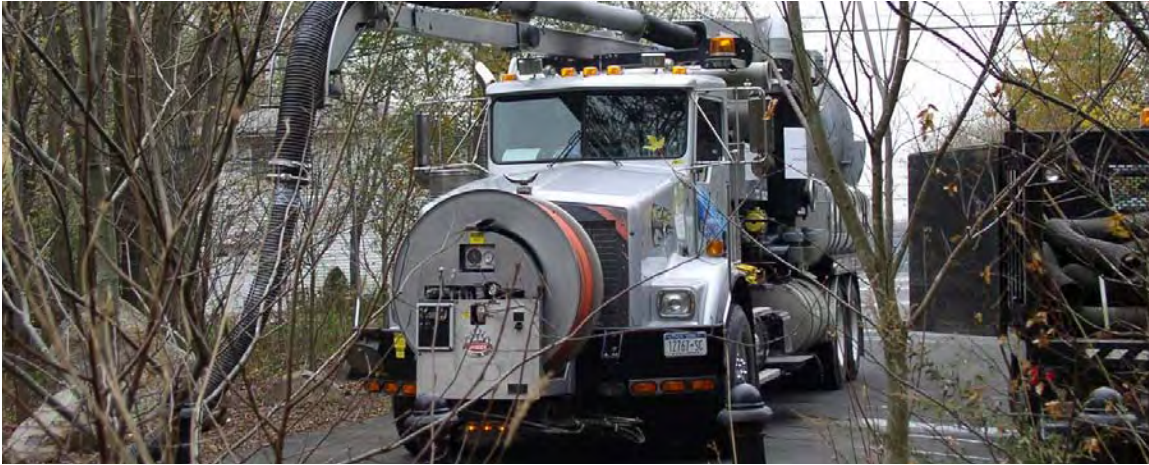
Figure 3-17: Sediment build-up in sumps should be removed using a vacuum or vector truck depending on the size of the system.
