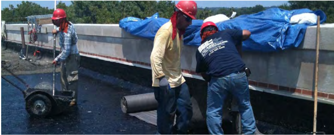
Figure 4-15: Application of tar and waterproofing membrane during installation of a green roof at PS118 in Queens.
