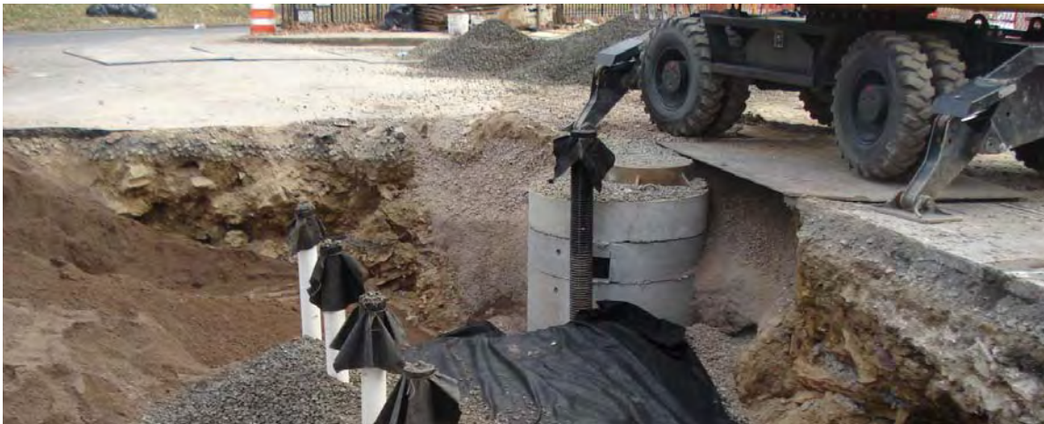
Figure 3-9: Observation wells allow property owners to observe water levels and flush the subsurface system should it become clogged.
