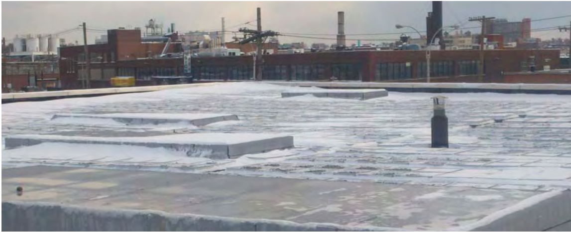
Figure 4-14: Blue roof system during winter installed at DEP's Storage Facility in Brooklyn. Prior to rain events, it may be necessary to clear ice and snow from around roof drains to allow for blue roofs to function properly during the winter.
