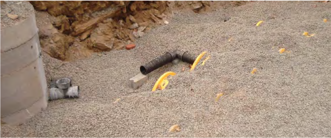
Figure 3-16: Embedment stone was placed over stormwater chambers at NYCHA's Bronx River Houses to provide structural support and additional storage volume.
