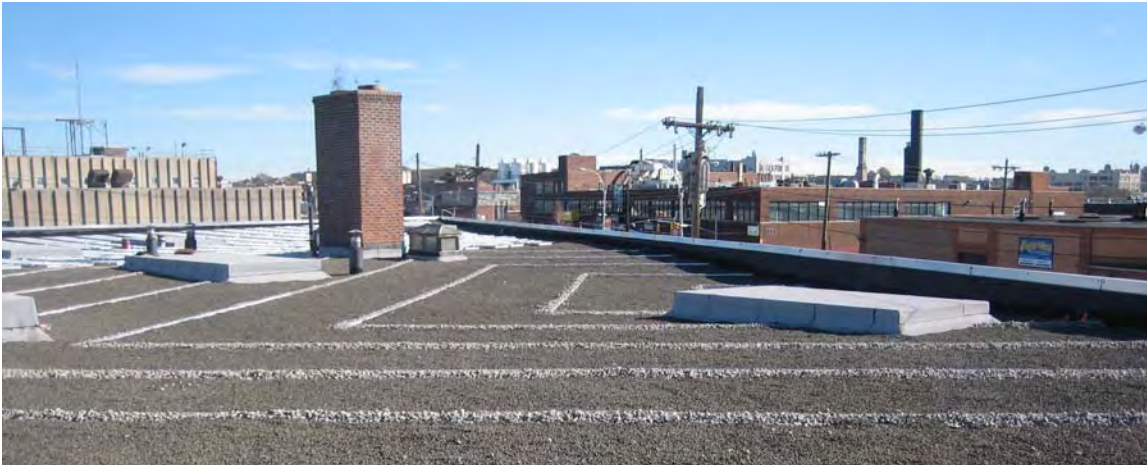
Figure 4-12: Intermediate check dams were installed on DEP’s Storage Facility in Brooklyn to control flow on sloped portions of the roof.
