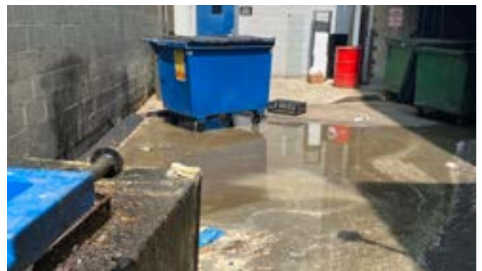
Mentor Way standing water problem in May 2023.
