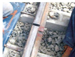
Figure 8.15: Gaps are left in railway tracks to compensate thermal expansion during hot season.
