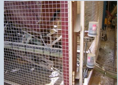
Memolubs on Tail drums and load chute – mounted behind guarding
