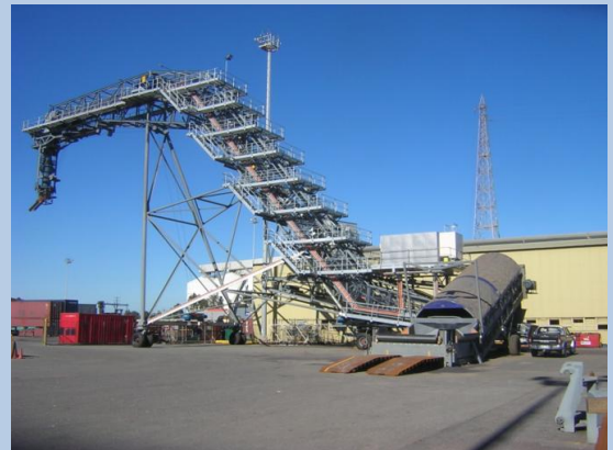
Ship loader – loads sand onto ships
